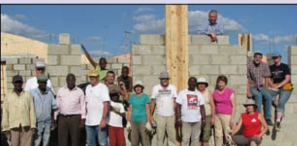
A Service and Learning team along with Duane (yellow hat), concrete masons and local children.
