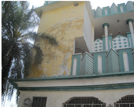
You can see the mark the water left on the second story of this home
