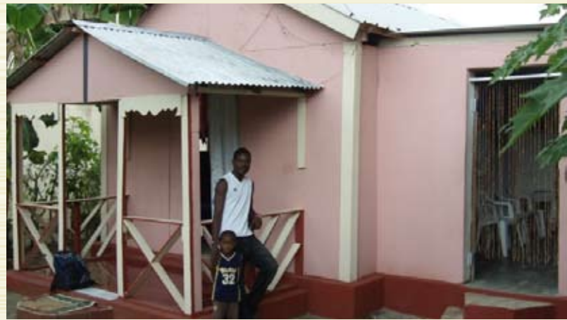
After home-owners laid the foundation for their new home, the components for CRWRC's wood-framed houses were delivered. Crews of Haitian workers then assembled the 2,500 houses to date.
